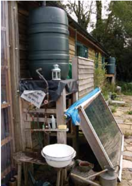
An excellent solar hot water system at Ourganics making full use of both gravity and the thermosyphon effect
