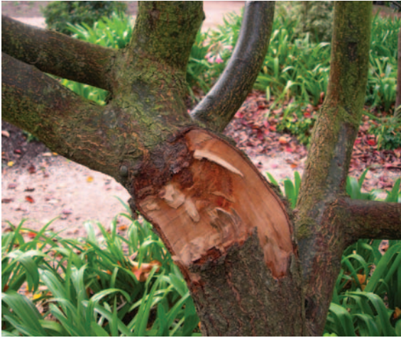
Figure 2.10 Too many branches originate from too small an area of trunk, even though some of the angles are wide and stable. Early pruning could have prevented this tragic result.
