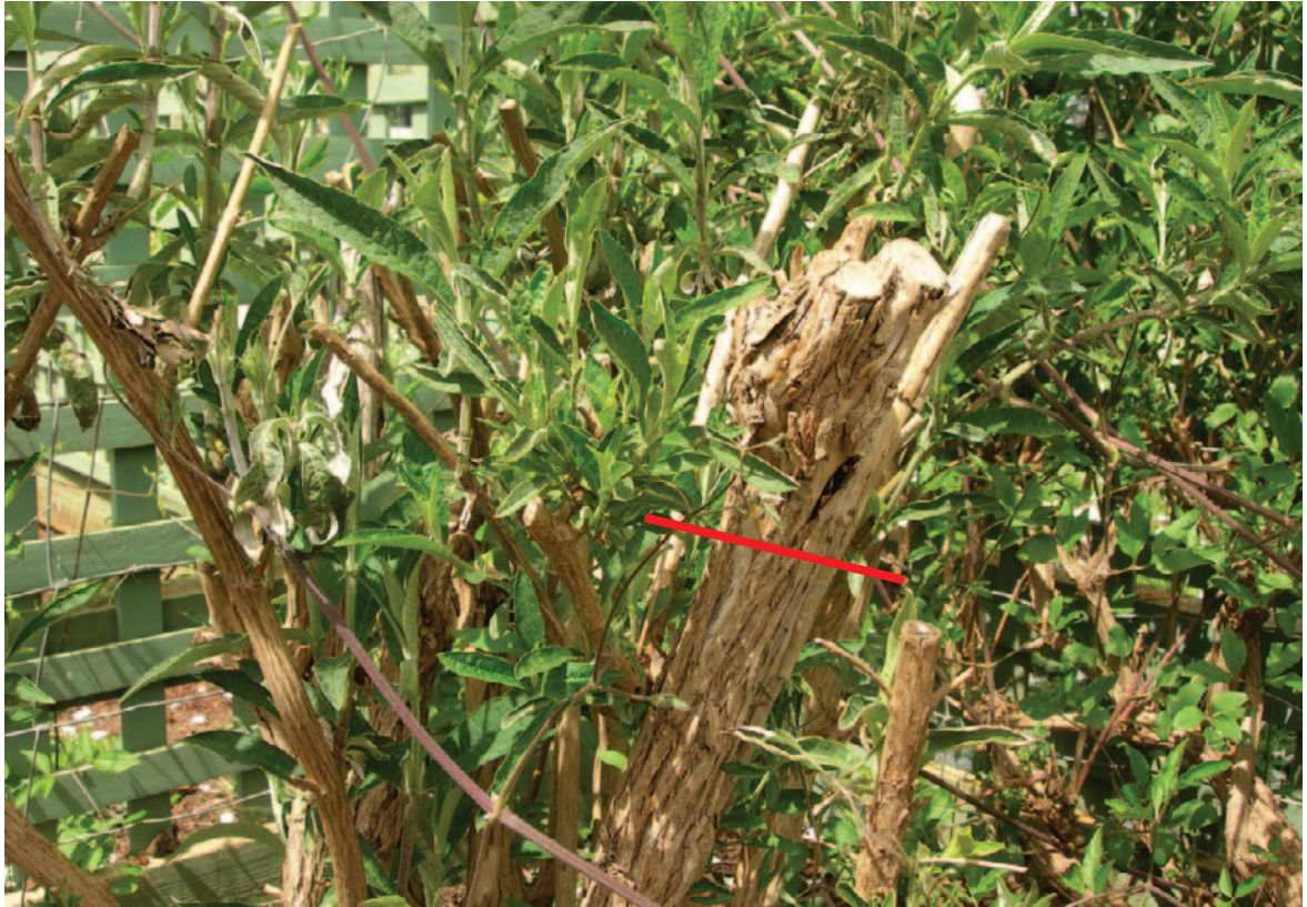
Figure 4.7 Note that most new growth is coming from the younger wood. Remove the crusty old wood to make room for new growth.
