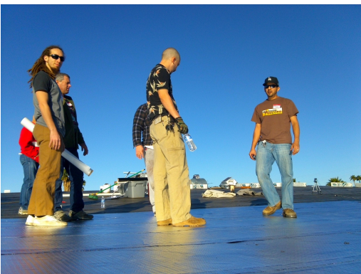
Dennis and a team of volunteers installing the peel and stick rolled aluminum roofing. Notice how reflective the surface is.
