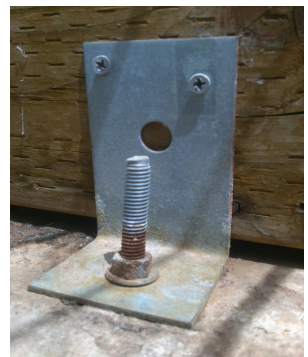
The frame of the GP is anchored to the concrete to prevent lifting in the wind.
