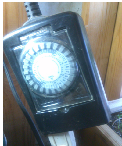
The indoor/outdoor mechanical electrical timer set to 30 on and 30 off for our aeroponic setup.
