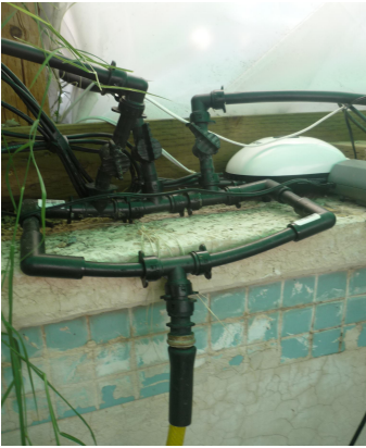
The water in the pond flows to the 3-way valve made from 1/2" irrigation tubing.
