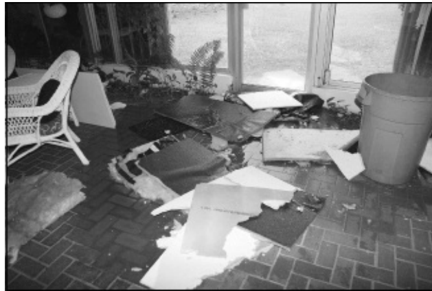
Interior damage caused by loss of roof covering during a hurricane. Photo by author.
