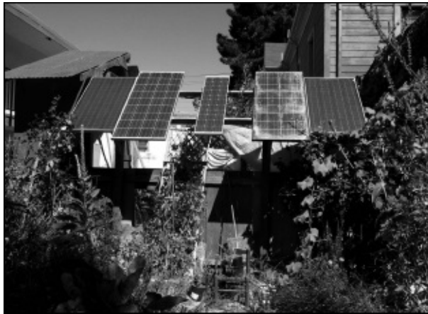
Recycled solar panels power outdoor garden lights and backyard stage at Mariposa Grove, Oakland, California.
