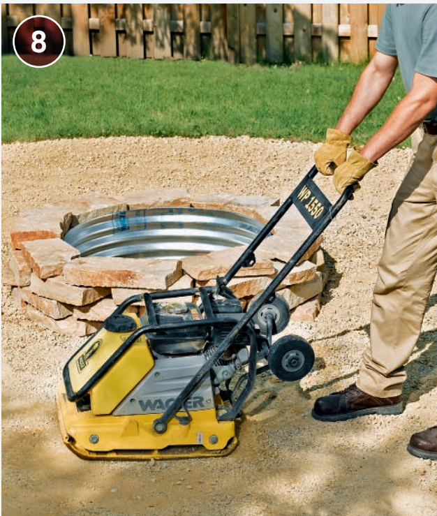
8 Compact the gravel in the seating/safety area using a rental plate vibrator.
