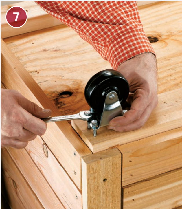
Attach the casters. Position each caster and drill pilot holes for each caster screw. Attach the casters with \frac{1}{4} \times 1\frac{1}{4} " lag screws.
