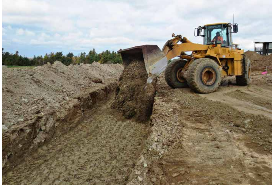
FIGURE 8.8. Clay being loaded into the keyway, 15 cm (6 in) at a time, then compacted.
