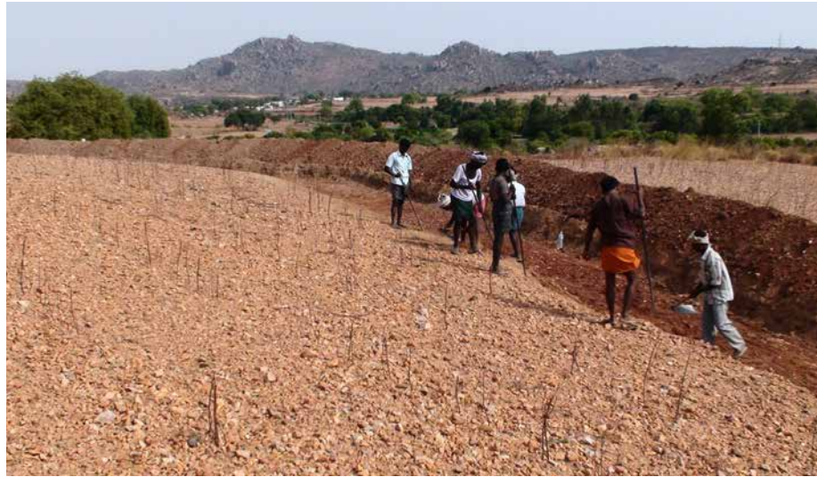
FIGURE 7.4. Workers groom the edges of the swale, using pikes to break through the hard soils.
