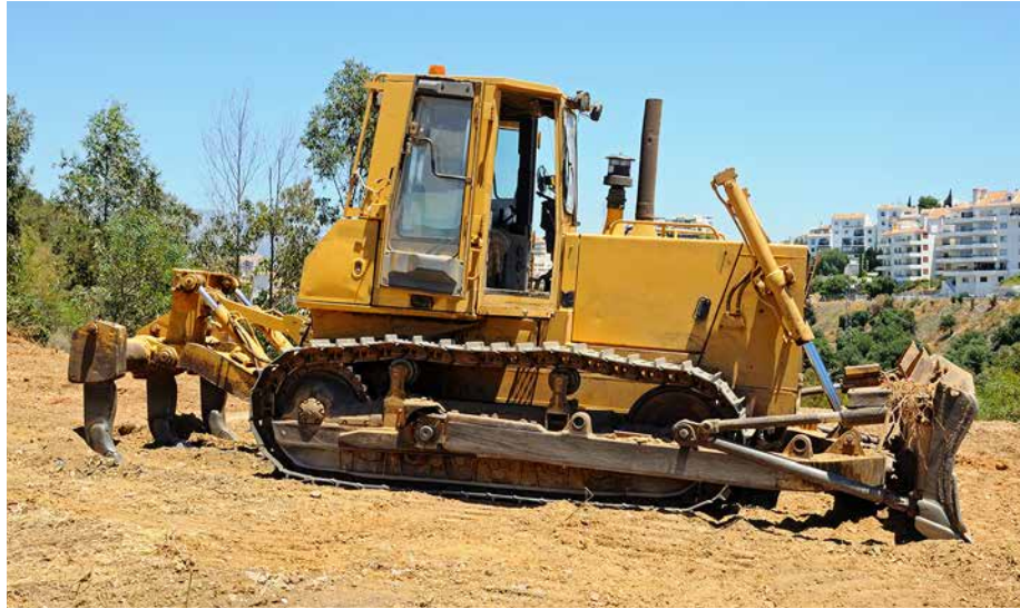
FIGURE 5.1. A bulldozer with VPAT blade (with straight blade attached) and rippers attached on the rear.
