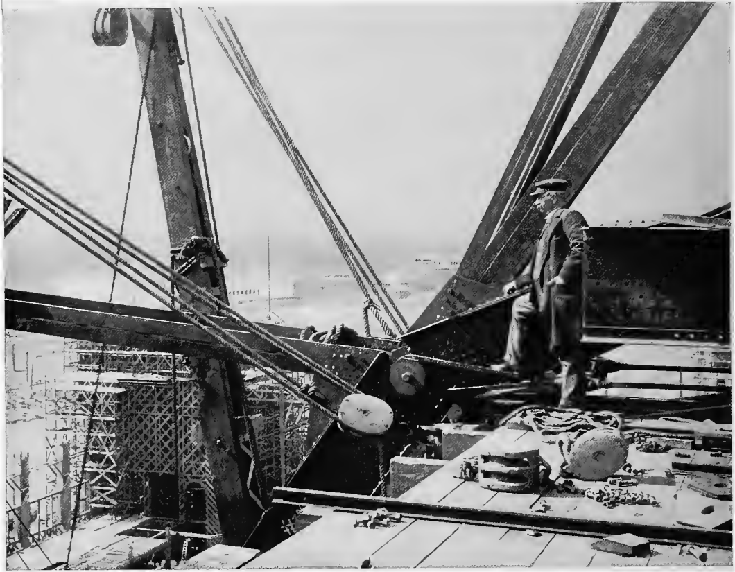
AN ARCH JOINT, 125 feet from the ground, in the Manufactures Building, April 10, 1892.
