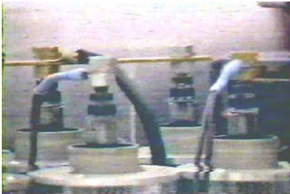
Ignitrons installed on the "Red Motor Cart"
